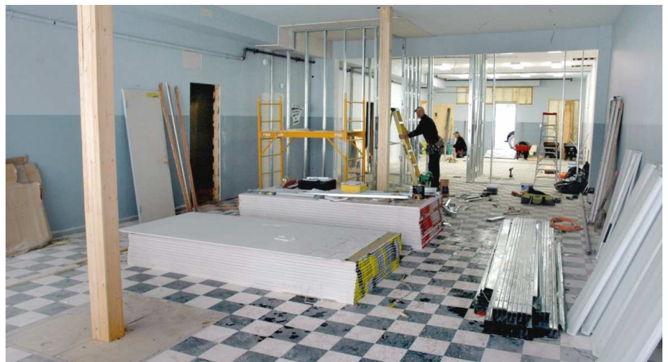
Major plumbing and ventilation upgrades are completed at the site of the L'Arche Café. Electrical contractors started their upgrades on October 31st, which is the final step before putting up the wall divisions and moving the Café furniture and equipment in. Please consult the Café page on L'Arche Winnipeg's website for opening date announcements.
