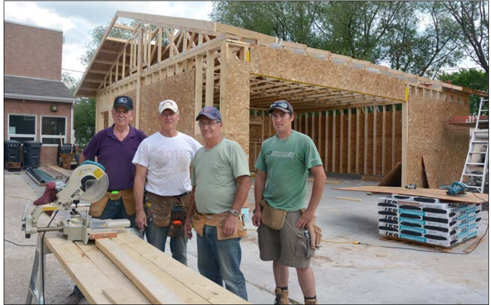
Part of the work crew building the garage: (l. to r.) Ron, Denis, Gerry, and Philip
